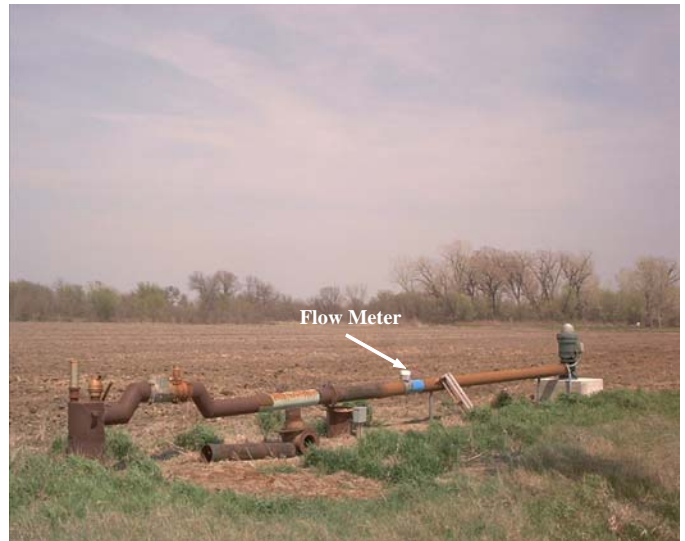
Acceptable Meter Installation
