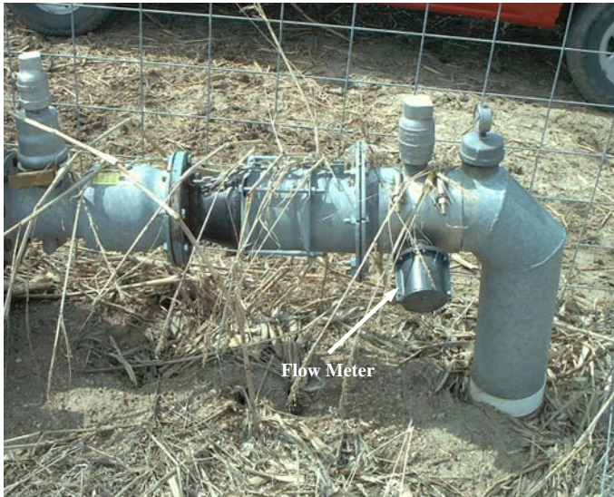
Unacceptable Meter Installation
