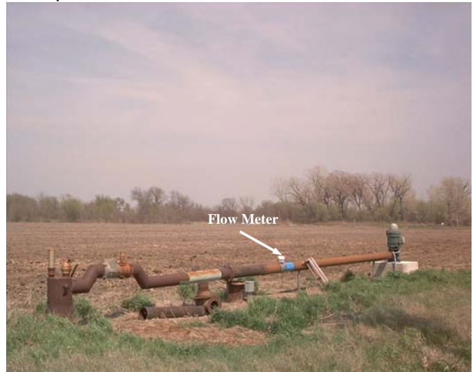
Acceptable Meter Installation
