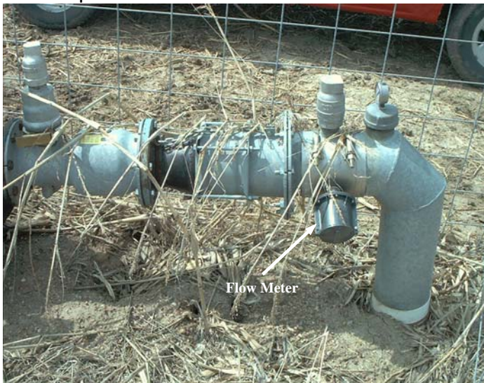
Unacceptable Meter Installation
