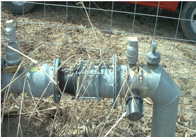
Unacceptable Meter Installation
