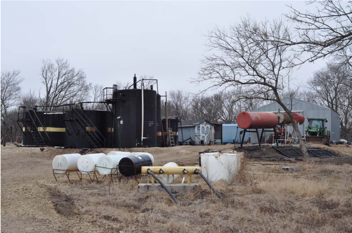
Photo of petroleum tanks in Kansas
