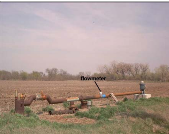
Acceptable meter installation
